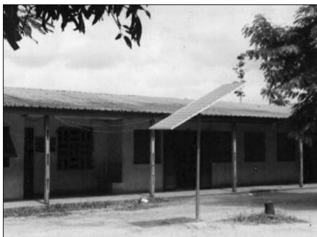
Photovoltaic panel for a primary school (Côte d'Ivoire).
