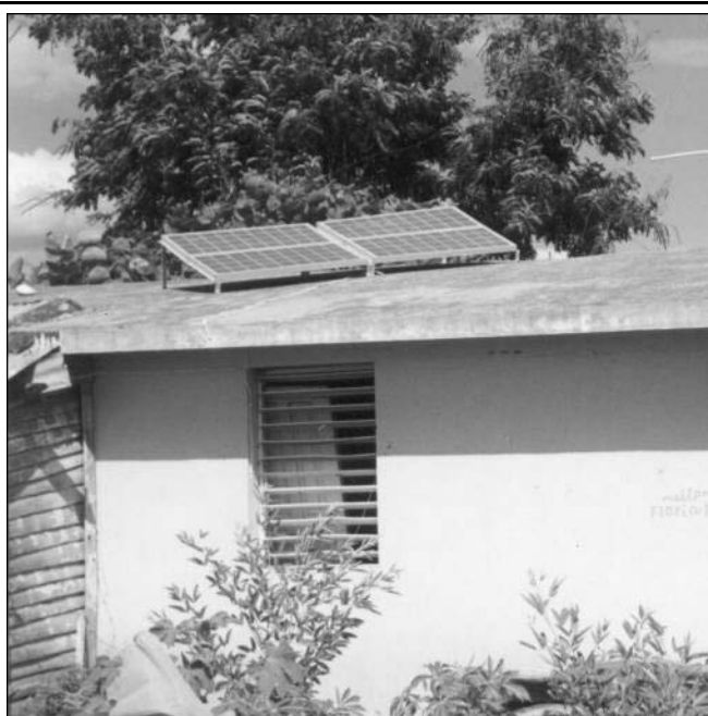
Solar photovoltaic panels installed on a school (Dominican Republic)
