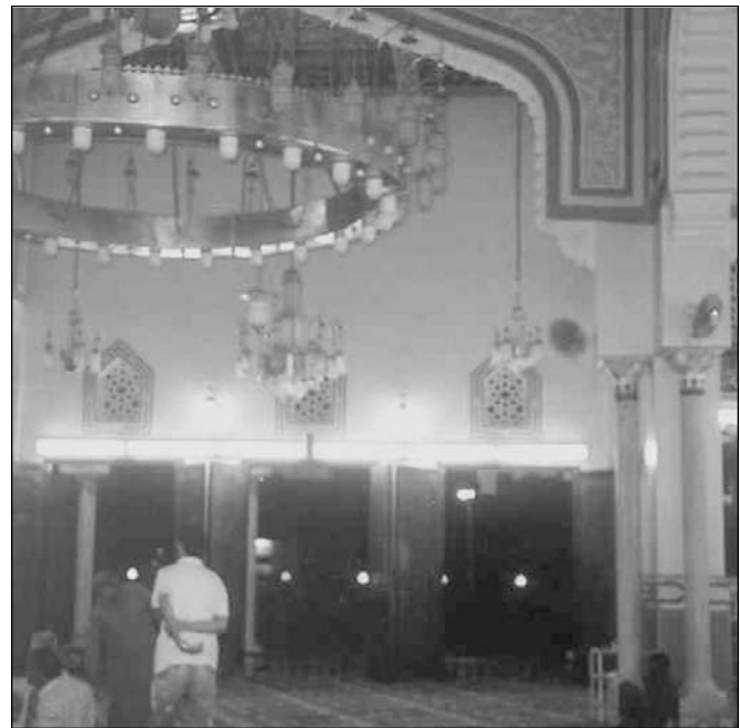
Energy efficient lighting installed and maintained by local youth (El Gharbia Governorate, Egypt).
