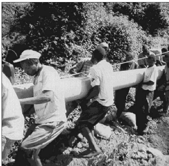
Tungu-Kabiri community working together to build a micro hydro power plant (Meru South District, Kenya).
