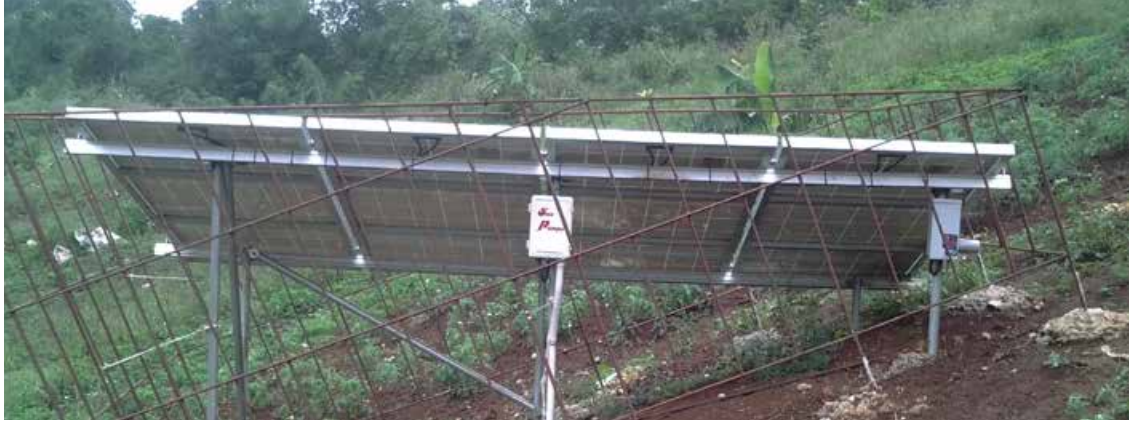
FIGURE 3: View of solar panels to provide electricity for the pump. Co-financing has been provided by Environmental Foundation of Jamaica .
