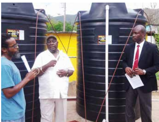
FIGURE 1: One of the refurbished community tanks with capacity of approximately 100,000 liters (58,000 gallons) has improved water availability for domestic purposes.
