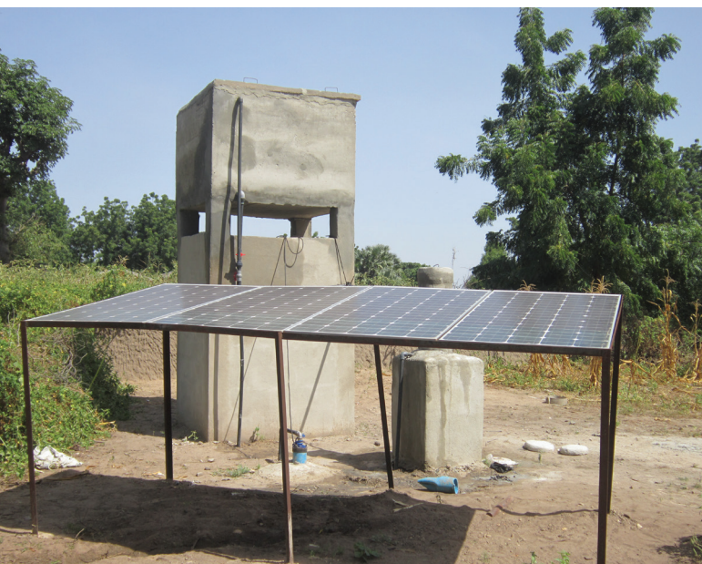
Photo 1a: Boreholes with solar powered pumps Photo credit: Hajara Haman (MBOSCUDA)
