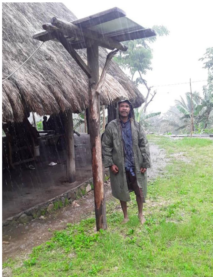
Fig. 5: Felipe Agustinho pictured with the installed solar panel at his Aimuti Uma-lulik. Datorua, 26/11/2022. Photo-Quintino Pires
