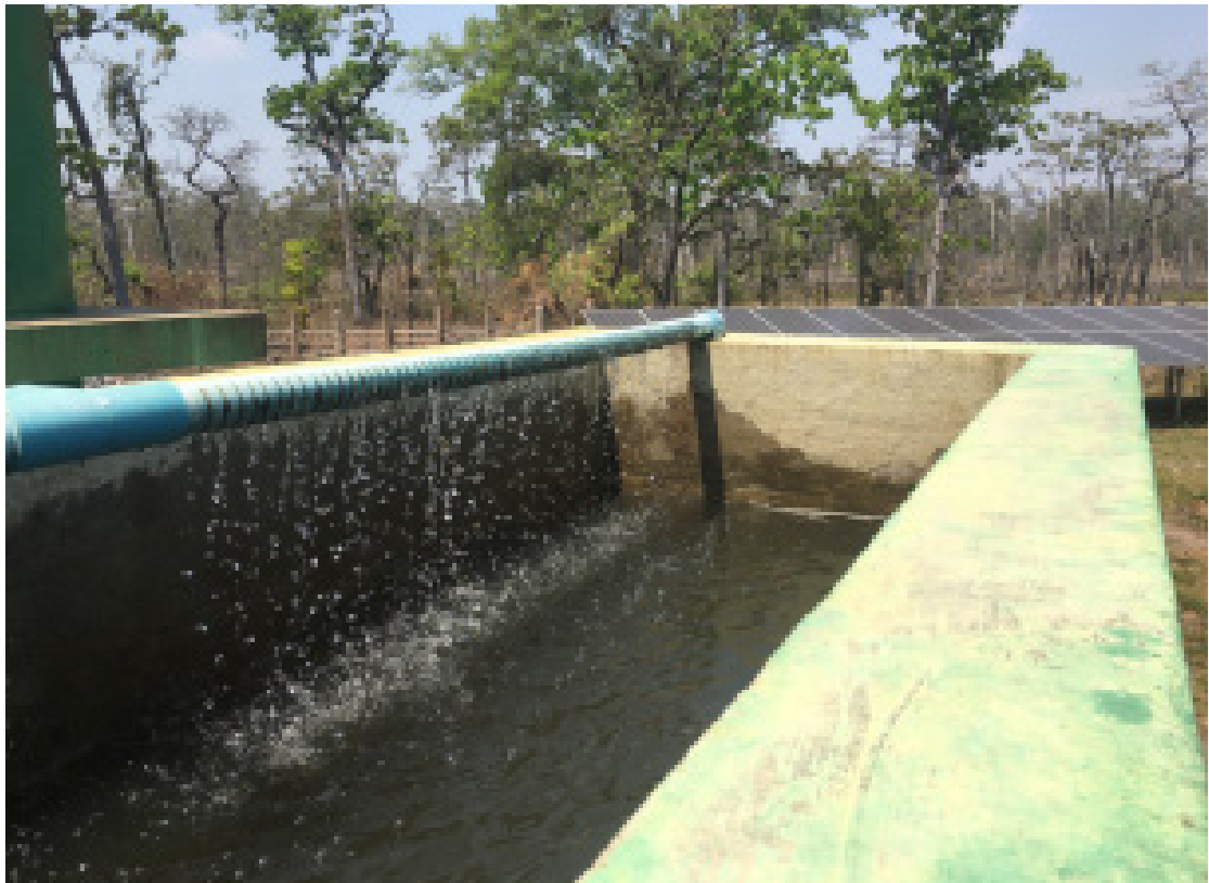
Water filtration tank
