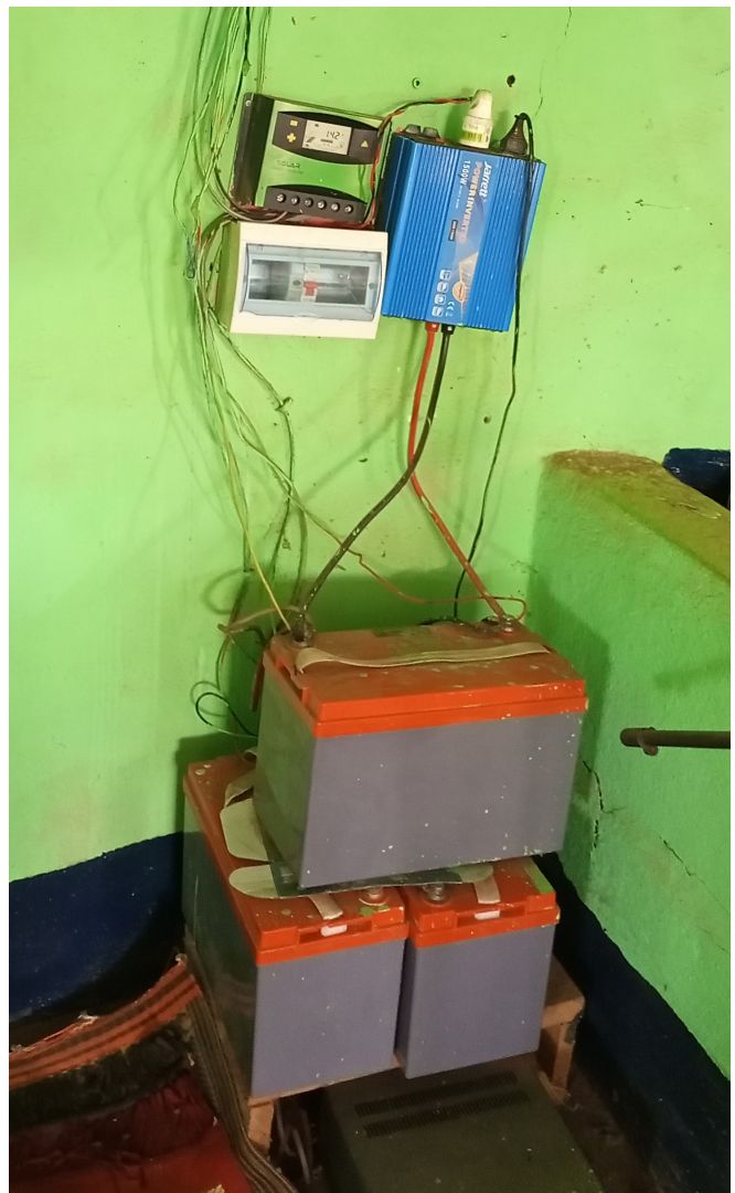
Photovoltaic system components at a mosque in Mobe
