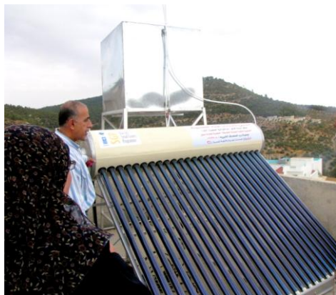
Solar powered water heaters
