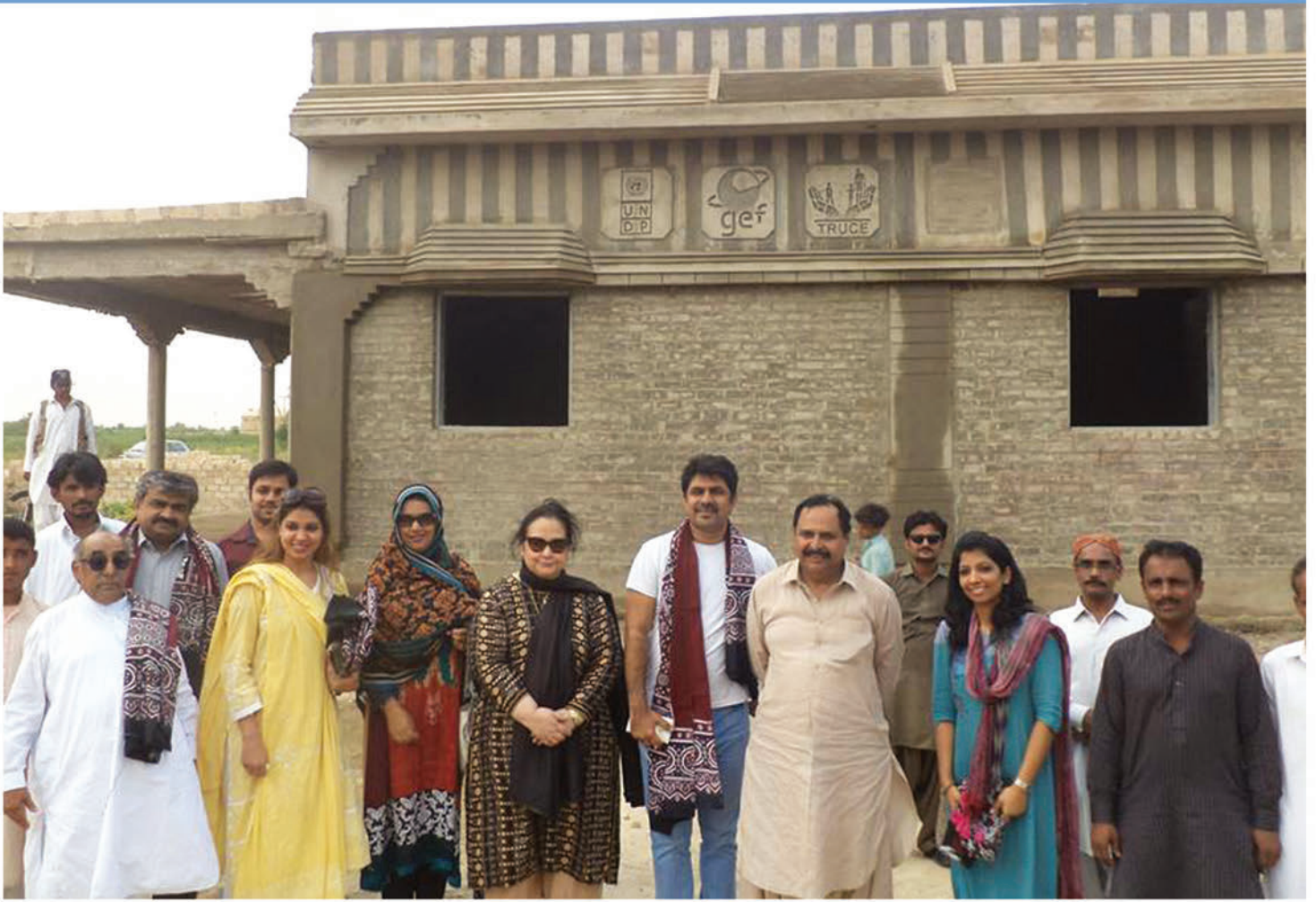
■ Federal Secretary Ministry of Climate Change Ms. Rukhsana Saleem visiting the under-construction UNDP-GEF SGP EE House Model
