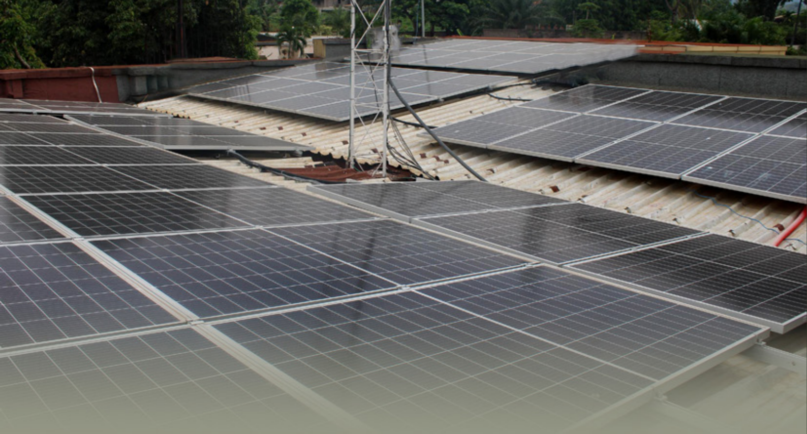
Partial view of the solar plant installed at the UNDP Cameroon Country Office to improve the organization's carbon footprint
