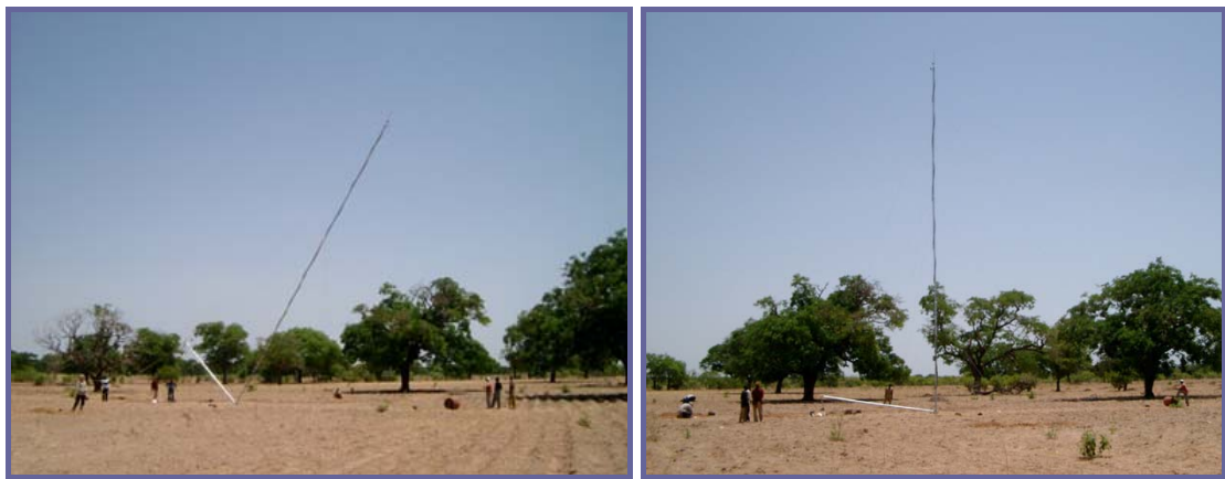
The 20m pole raised at an angle of 45°, with an electric winch (left) ; The pole is raised to vertical (right).
