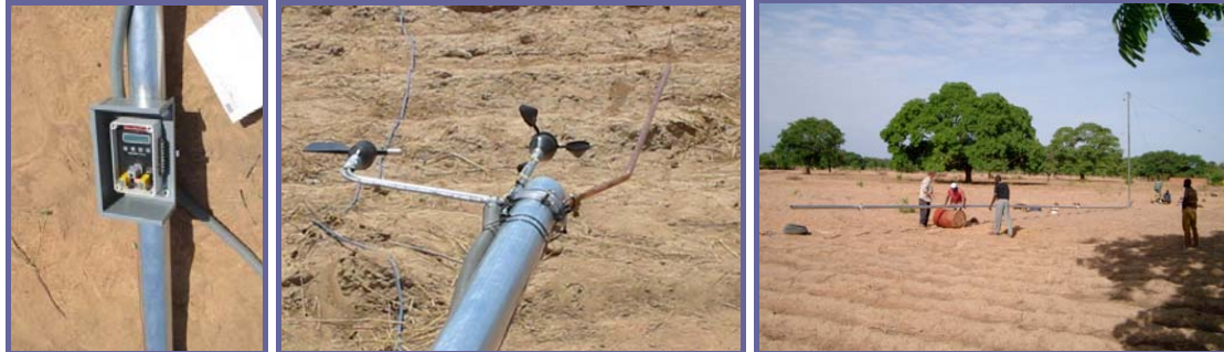
Data recording box (left); The Sensor of wind direction and the anemometer (middle); Assembling of the Gin-pole (right).
